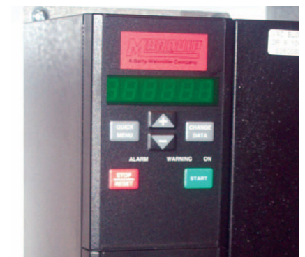
Variable drive for blower motor
